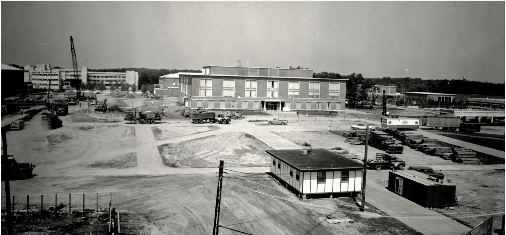
Construction on the Stony Brook Campus, c. 1967. Pictured center: the Library. Pictured left, in the background: Earth and Space Sciences building.
